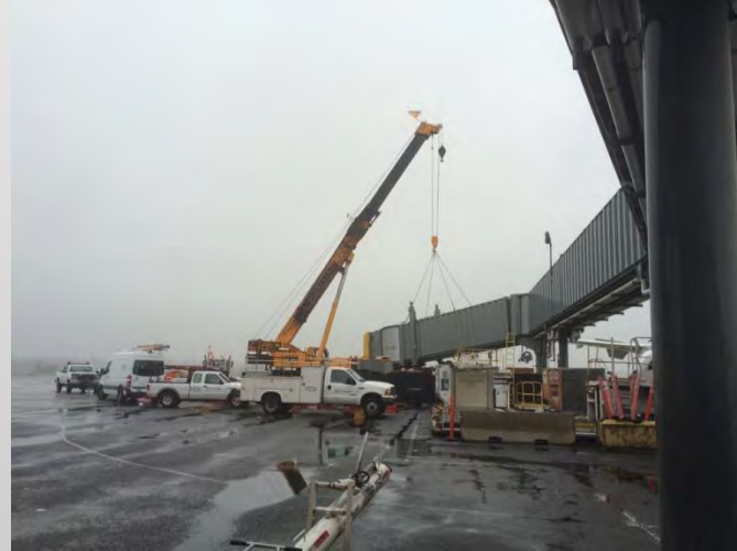
Passenger Loading Bridge – Gate S15
