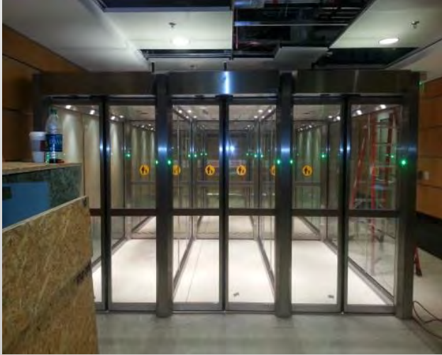
Security Exit Lane Breach Control
