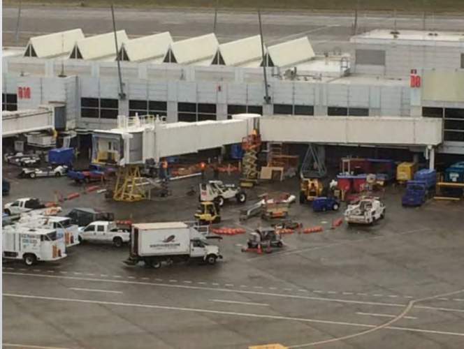
Passenger Loading Bridge – Gate B8
